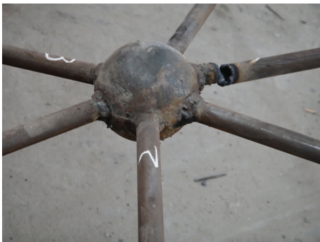
图 6 损伤杆件 Fig. 6 Damaged member
